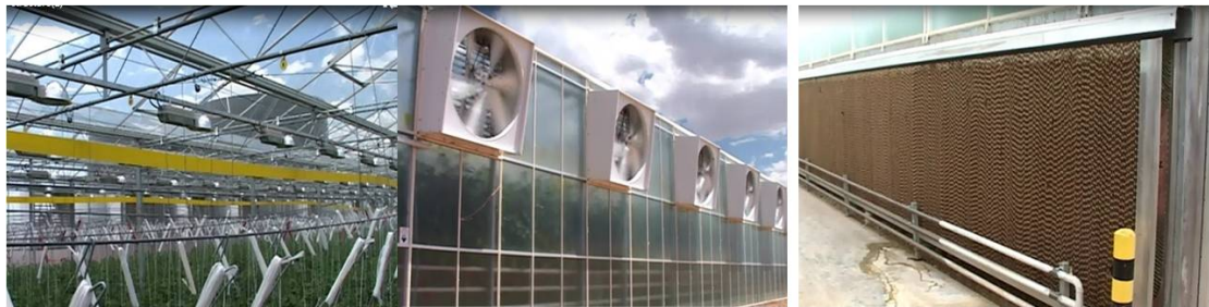
(the greenhouse's roof and cooling system)
