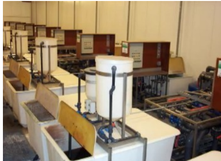
(Silos collecting water)
